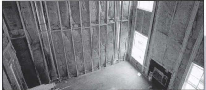
For homes built on a concrete slab, rigid foam board insulation should be installed around the perimeter of the slab.
