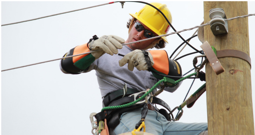
Pictured above: CFEMC's Noah Watson competing in the 2023 Georgia Lineman's Rodeo. Pictured right: Lineworker apprentices and journeymen from across the state participate in the opening ceremony for the 2023 Georgia Lineman's Rodeo.
